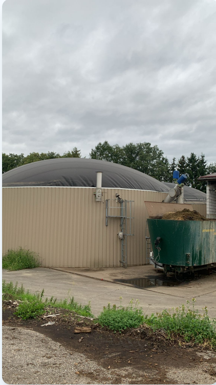
Digesters and feed mixer
